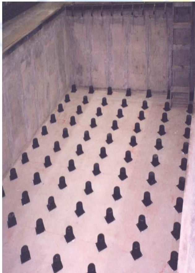
(Fig: 27- Isolators positioned on pit floor prior to forming the foundation above)
